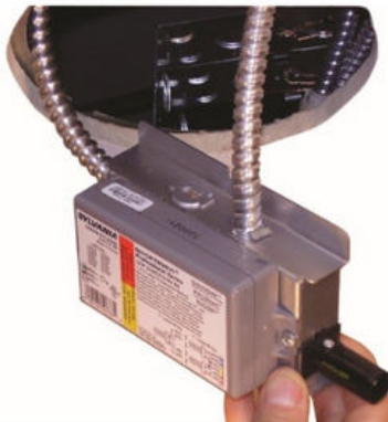
Fig. 39 Inner junction box cover (3D Cover #1242-18B) with mounted driver, removed for servicing below ceiling
