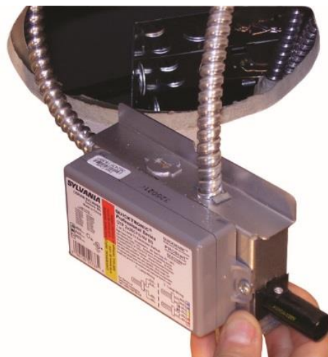
Fig. 35 Inner junction box cover (3D Cover #1242-18B) with mounted driver, removed for servicing below ceiling
