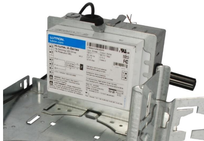
Fig. 34 Driver affixed to outside face of Inner junction box cover (1242-18), mounted to junction box 1232
